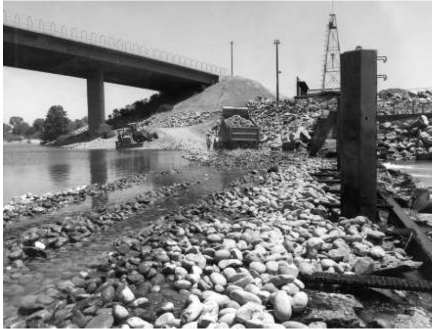
Figure 3-17 Rock fill being placed upstream of fish weir to facilitate repair. 8/3/82 D.M. Westphal, Photo (Bureau of Reclamation).
