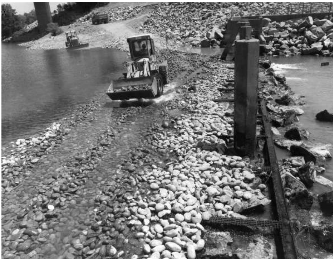
Figure 1-14 Repair of the fish diversion structure at Nimbus Fish Hatchery (photo: D.M. Westphal, Bureau of Reclamation, 8/3/1982)
